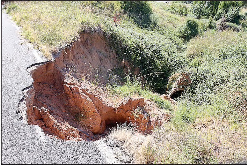
No repairs have been undertaken at this landslide near Old Tallangatta.
