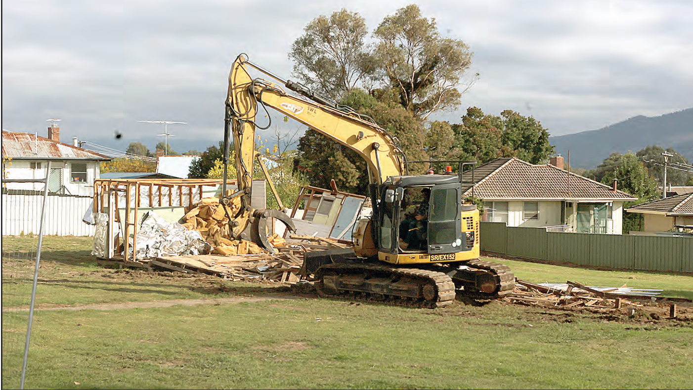
The former Guides Hall has been demolished to make way for a new food service facility.
