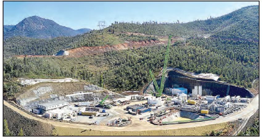
Talbingo adit, where TBM Lady Eileen Hudson is being reassembled for excavation of the tailrace tunnel.
