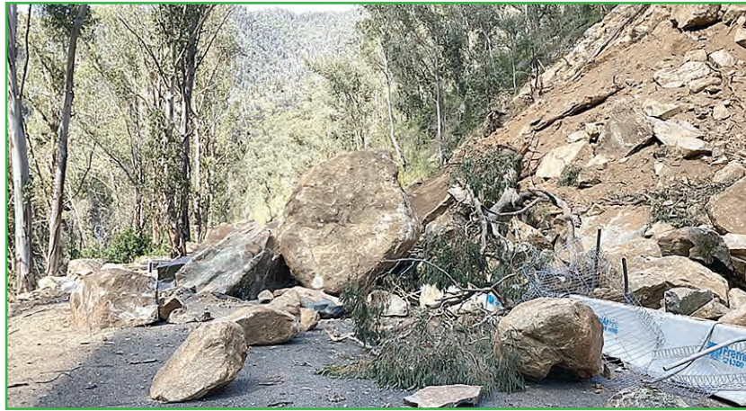
Several landslides have kept the Elliott Way closed since August last year.
