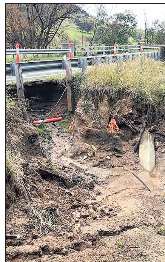
The washaway on the north side of Granya.
