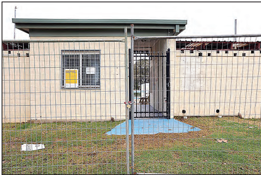
Work has started on replacing the old amenities area at the pool.
